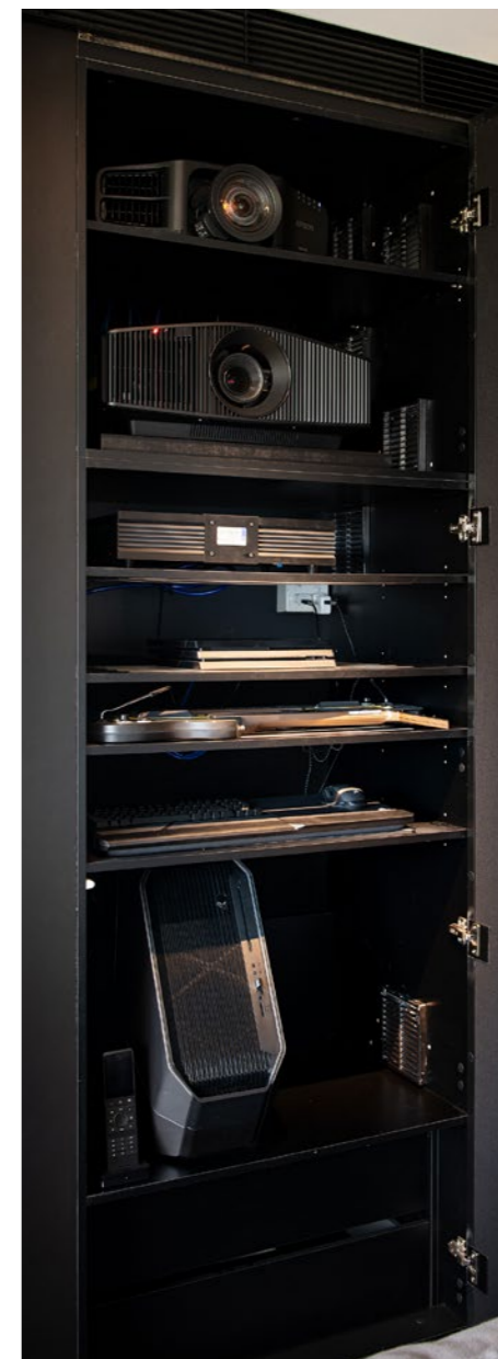
◀ The seats were positioned to provide even bass response, and then calibrated to deliver the flattest frequency response. Note also how neatly the rear wall incorporates the projection ‘hush boxes’ and cabinetry (above), all of which is actively cooled to ensure optimal operation of all electronics.
